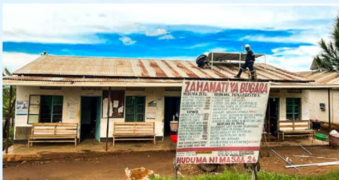
Bugara dispensary is one of the 107 health facilities MDH has supported with installation of solar panels to ensure uninterrupted power supply for sustainable continuity of health care services.
